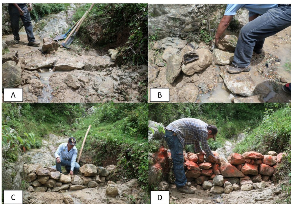
Figure 3. Procedure for building a dam with arranged stone: A) Layout, B) Embedding in the bed and margins of the gully, C) Placement and arrangement of stones that make up the body of the work, D) Construction of the apron and spillway of the dam.
